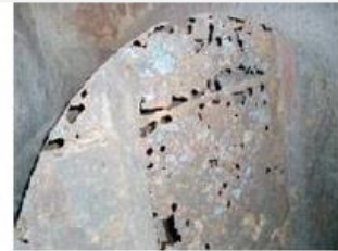
Holes / heavy corrosion on damper housing and flaps
