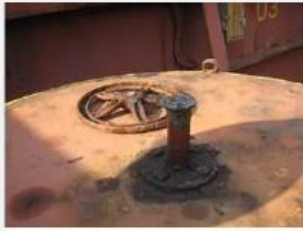
Operating handles not in good working condition
